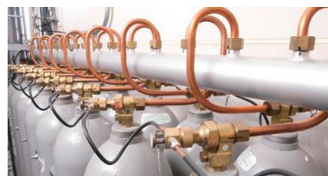
Gas-based fire extinguishing systems
