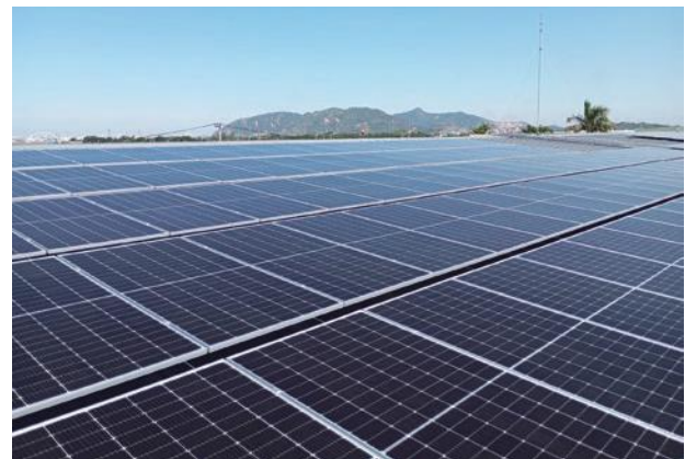
Solar panels on factory roof (TPT)
