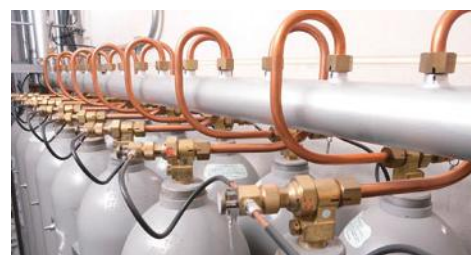
Gas-based fire extinguishing systems
