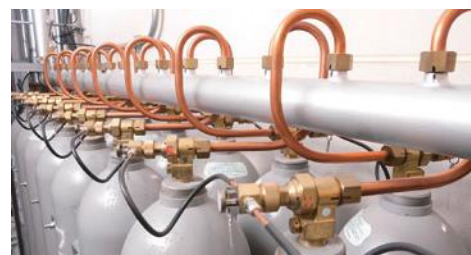
Gas-based fire extinguishing systems
